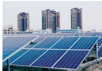
Solar power panels installed on the roof
